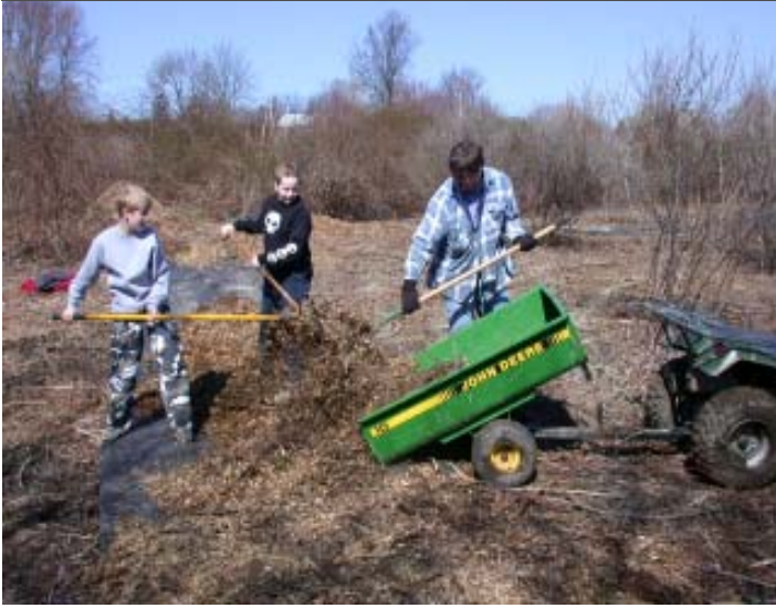
Justin DeFrank and Conor Hesse help Justin's father, Kevin, unload a cartload of woodchips onto fabric covered pathways between the Elk Ridge and Nottingham Schools. They were among 30 volunteers who helped to finish Phase I of the Oxford Wetlands Project on March 23. Story on page 2.
